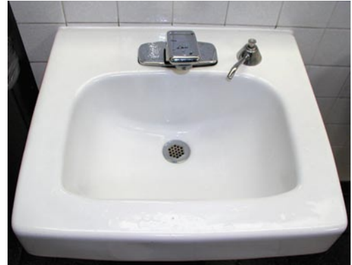
One of many automatic shut-off faucets the Airport uses to conserve water.
