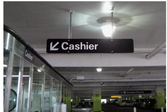
Energy Saving Fluorescent Light in use in Garage G.
