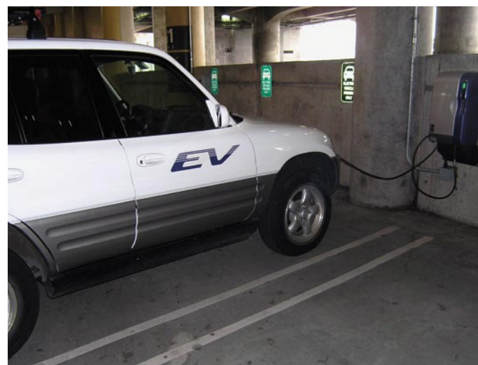
One of three electric vehicle recharging units available for public use in International Garage G.
