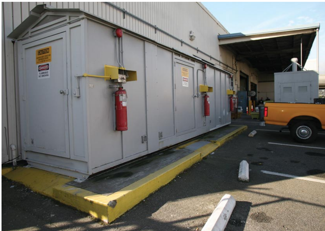
Containment trailer with controlled access and fire protection equipment safely stores hazardous materials.
